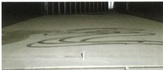
Ventilation ductwork before cleaning
