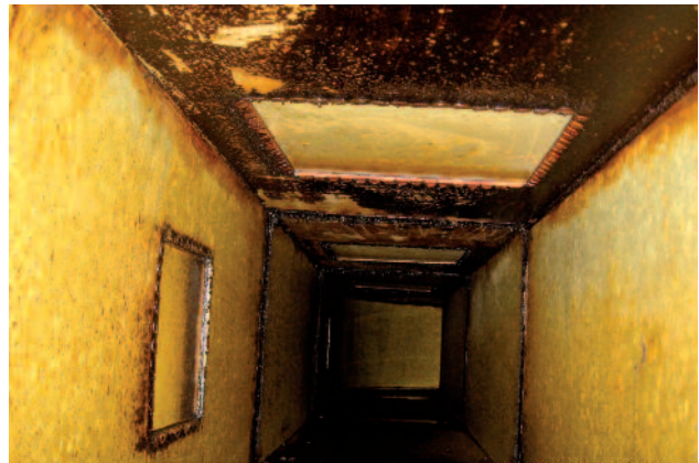
Kitchen extract duct before cleaning
